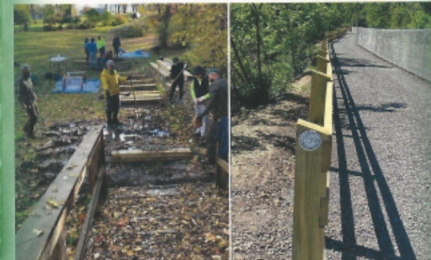
Fish Creek boardwalk work party Newly open Auburn section by Victor Insulator
